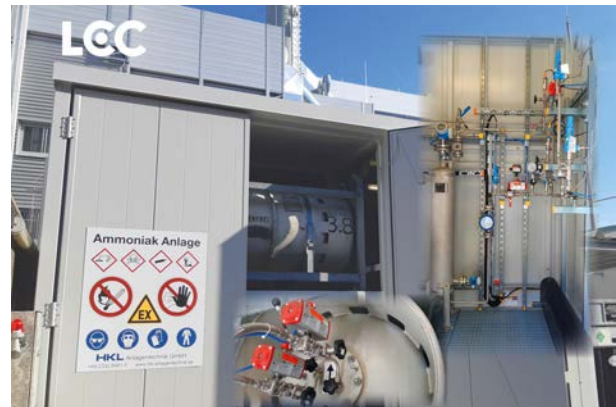
Figure 1: Ammonia storage in a mobile container
